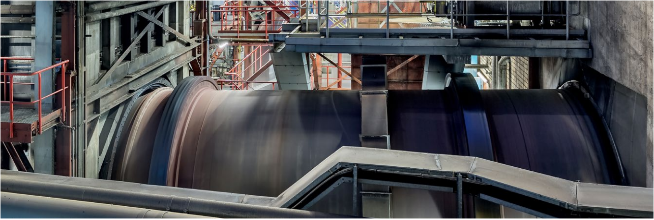
Hazardous waste treatment, AGR Group, Herten, Germany
