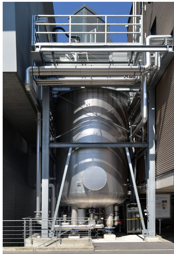
BiON ® technology, methanation reactor
